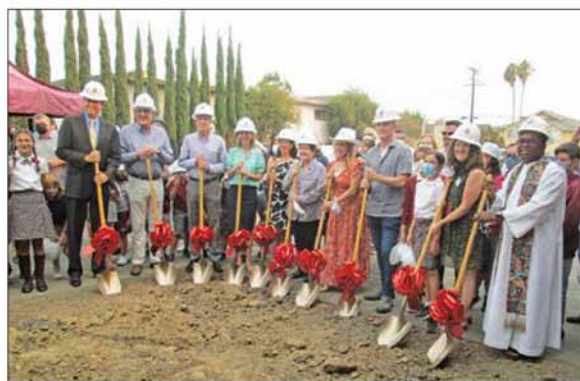
Mayor Katherine Lee joins church and school dignitaries for groundbreaking for the new All Souls language building.
